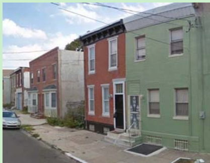
The green home does not maintain the same size/ scaled fenestration as its neighbors.
