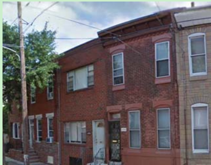
The center left home has windows replaced with windows that are incompatible with windows in Point Breeze.
